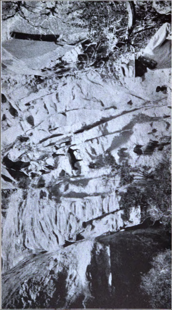
The packtrain's final and successful passage of the divide of Red Bud Pass. Note the tilted rock masses in the centre. The centre one was blasted partially, while that on the left was blasted off entirely.
