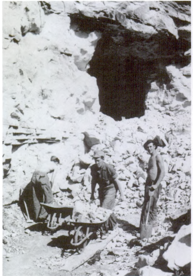
Figure 4.10. Workers remove blast rubble from coyote hole or pilot bore in one of the road's three tunnels. Colorado National Monument Museum and Archive Collection. ▶ ▶ ▶
